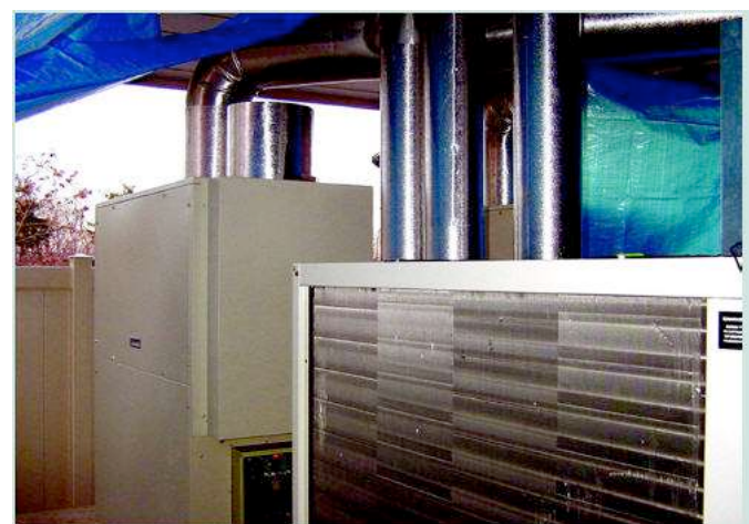
Figure 4: Microturbine and exhaust-driven air conditioner.
