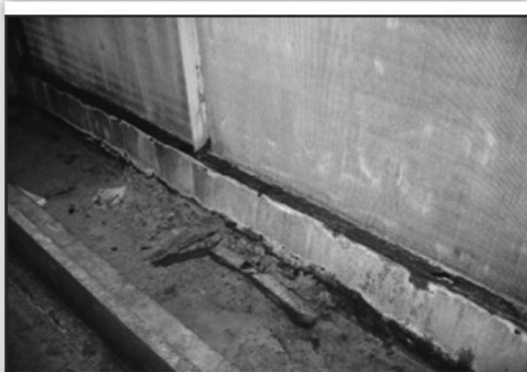
HVAC unit corrosion (Controlled Release Technologies)
