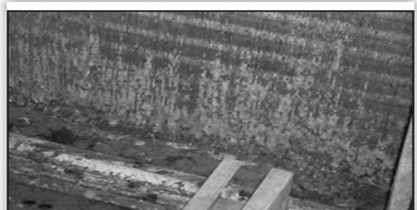
Fouled HVAC cooling coil (Controlled Release Technologies)
