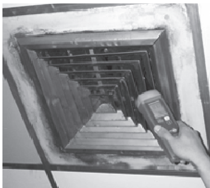
Figure6 “Mold on air diffuser and ceiling”
