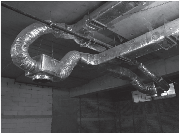
Figure10. Air diffuser with both re-circulated air and treated outdoor air supply
