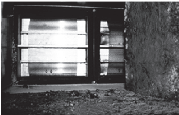
Figure5 “Mold in the Air Plenum”
